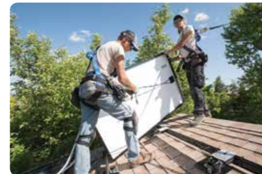
SolarEdge at home
