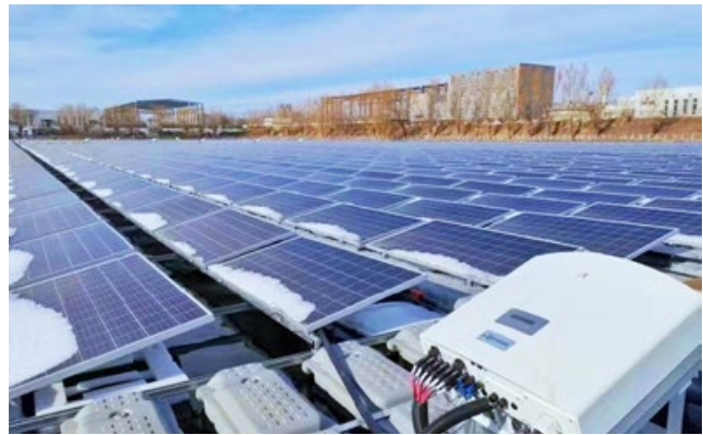
Beijing Shunzhen Green Harbor's Plant 5.5MW
