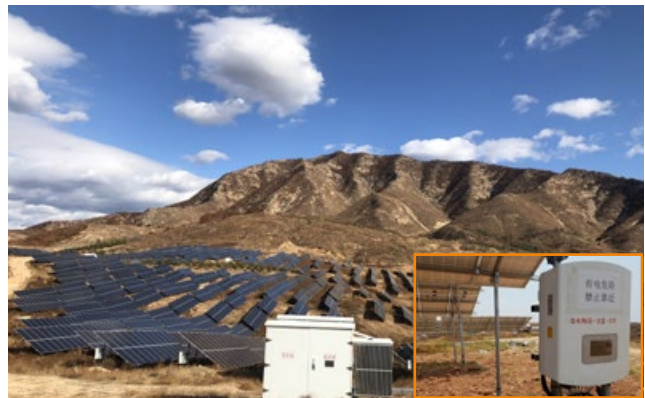
Liaoning Gaizhou Jiuzhai PV plant 20MW
