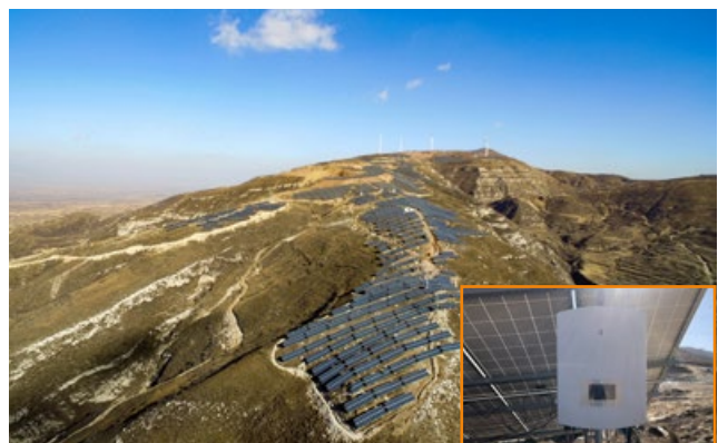
Shanxi Xinzhou NingWu poverty alleviation PV Plant 18.11MW
