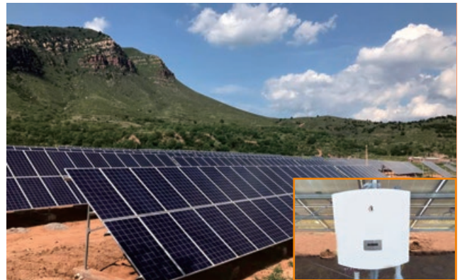
Shanxi Xiyang poverty alleviation PV Plant 7.2MW
