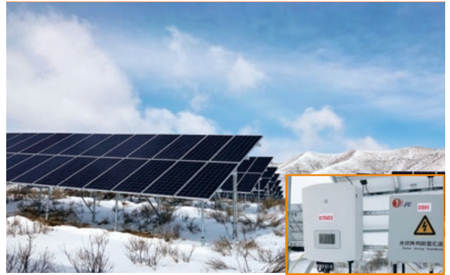
Shanxi Guangling PV plant 1.47MW
