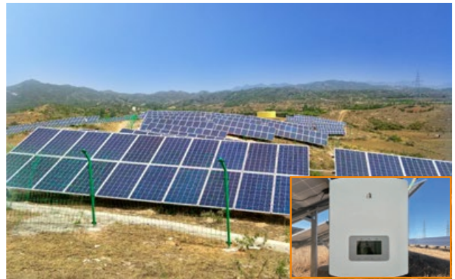
Hebei Qinghuangdao poverty alleviation PV Plant 9.7MW
