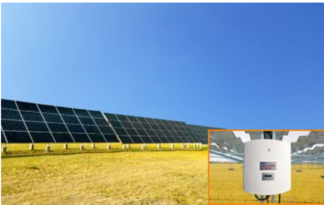
Huaneng Yimin surface mine PV plant 20MW
