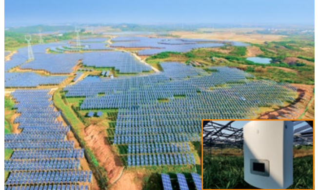
Zhejiang Hangbu Agricultural-photovoltaic hybrid PV plant 30MW
