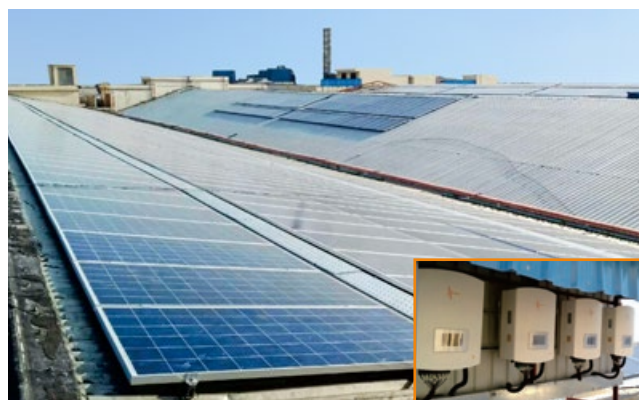
RSWM, India 3.6MW
