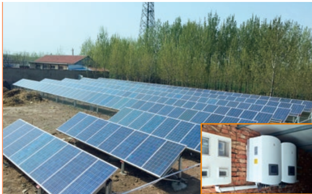
Shandong Leling poverty alleviation PV Plant 50kW
