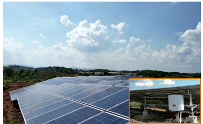
Jiangxi Ganzhou PV Plant 3.5MW
