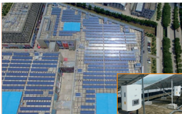
Ninghai AB hall, modern home plaza 1.53MW
