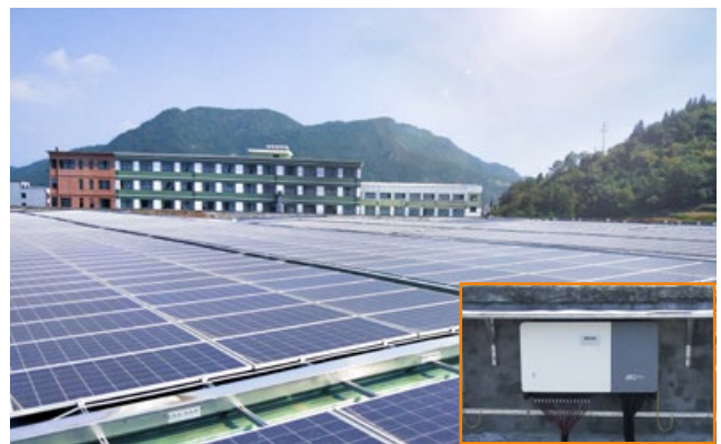
Tyco Electric, Panan Jinhua Zhejiang 1.5MW
