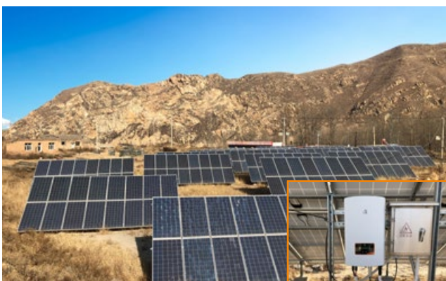
Shanxi Xinzhou FanShi poverty alleviation PV Plant 8MW
