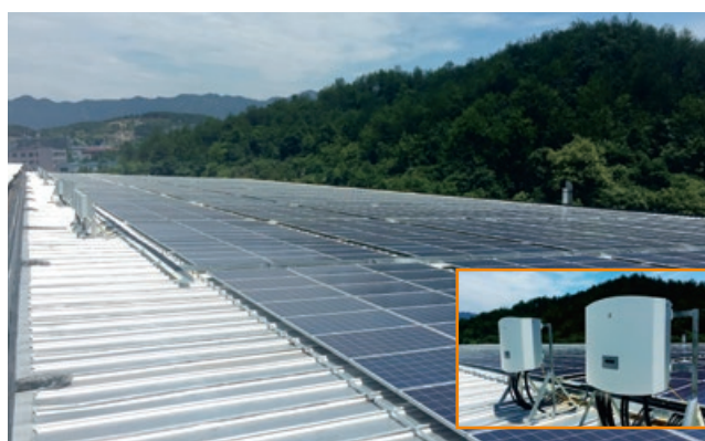
Hainan JiuLongGlass 1.7MW
