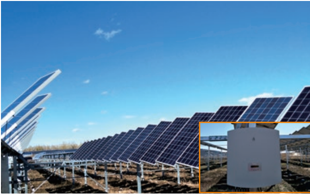
Hebei Zhangbei Agricultural-photovoltaic hybrid PV plant 50MW
